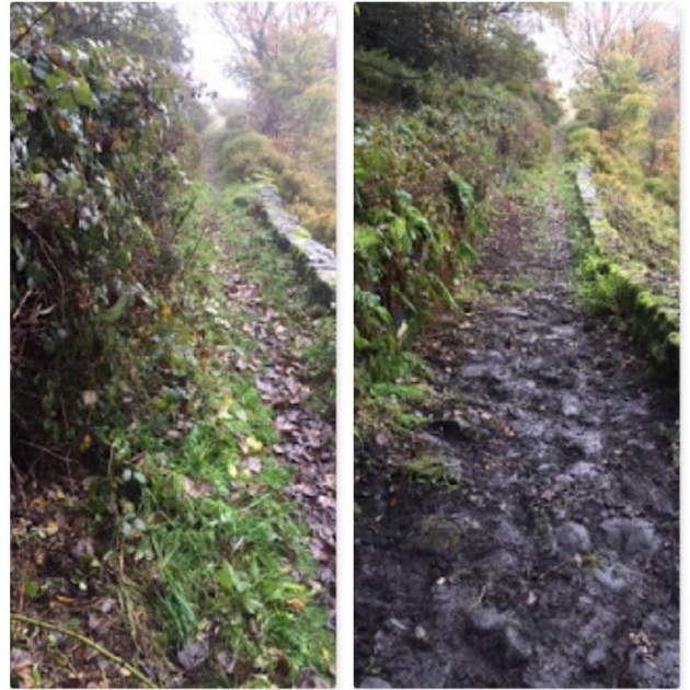
Todmorden 'There and Back' routes were all refurbished – including cutting back and path widening (before and after photo)
