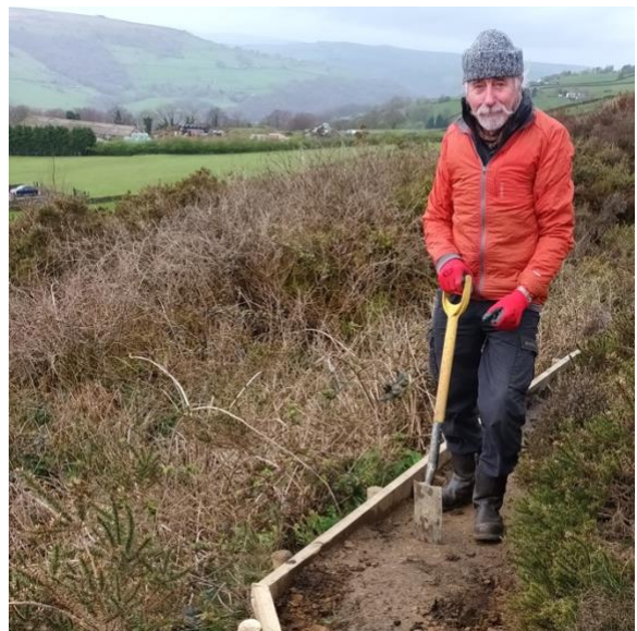
Smart revetments on Midgley Moor.
